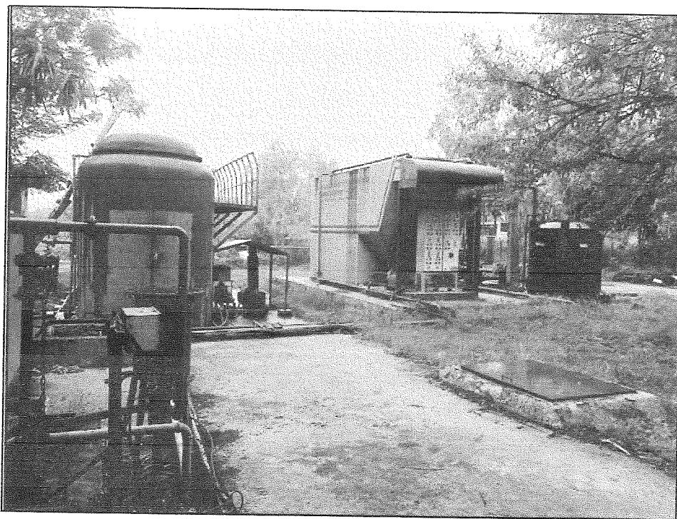
Photographs of the Sewerage Treatment Plant (STP) provided within project premises
